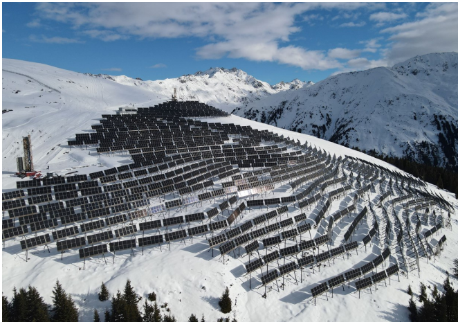
Winter power: before weather interrupted construction, 20 per cent of the installation had already been connected to the grid.
